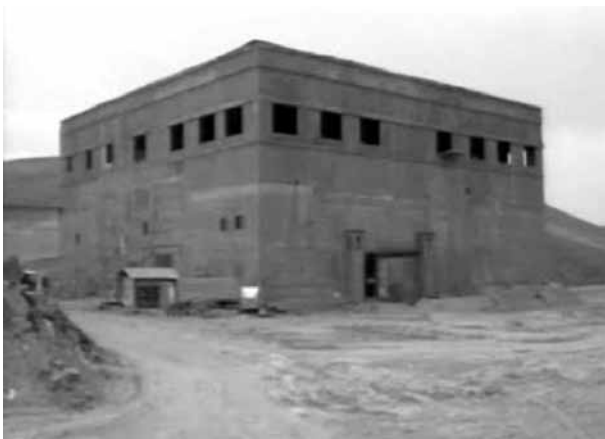
Image of a suspected Syrian nuclear reactor under construction with North Korean assistance from an April 24, 2008 Central Intelligence Agency (CIA) video. Israel destroyed the facility in September 2007, and Syria has not cooperated with an IAEA investigation about its possible role in a Syrian nuclear weapons effort.
